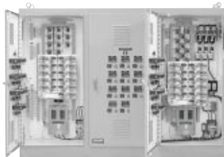
Custom Panels & Control Systems
